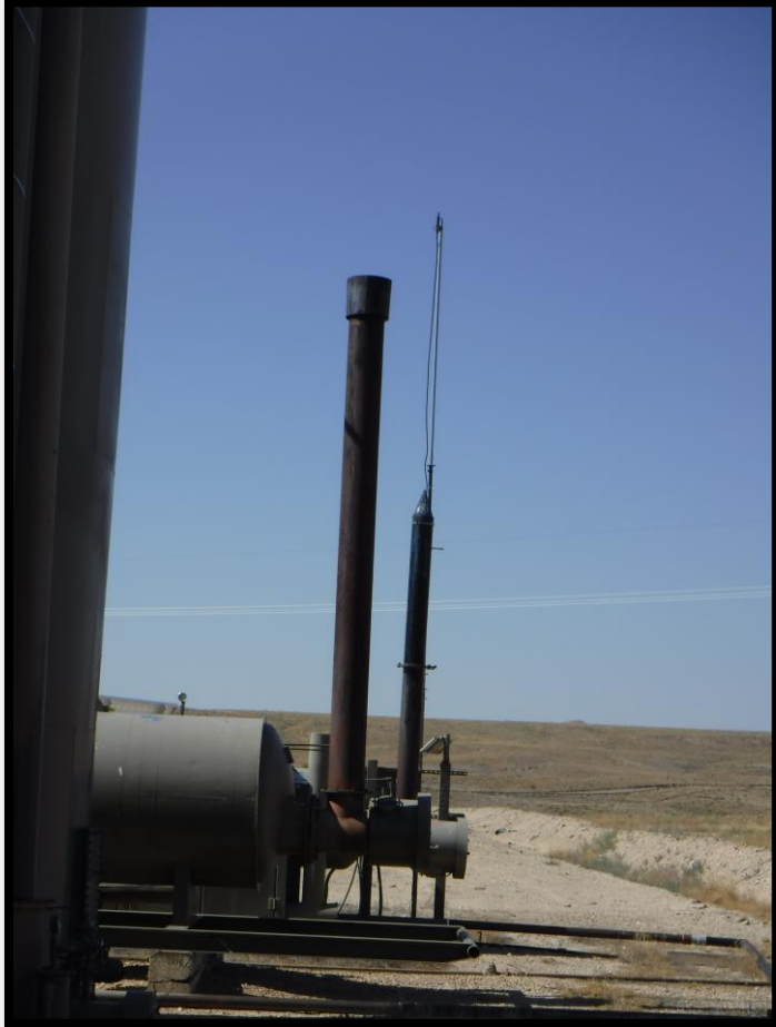
Exhaust stack is missing anti-perch device
