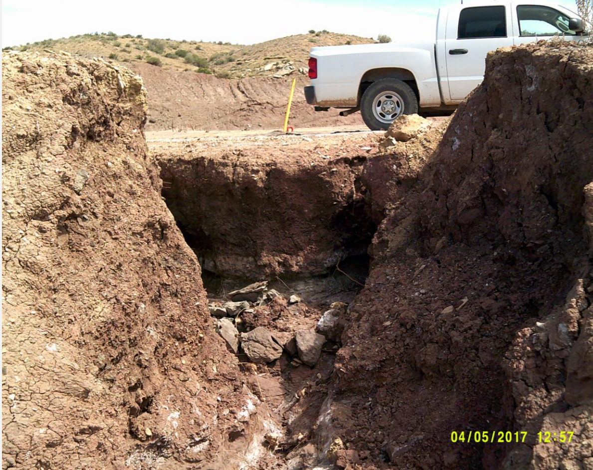
Erosion and channeling off access road
