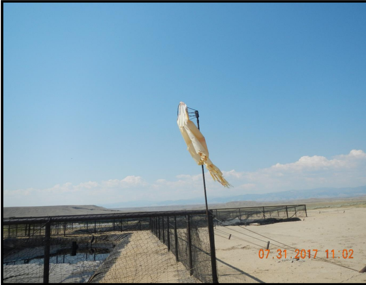
Windsock in bad condition on H2S location; No other wind indicators present
