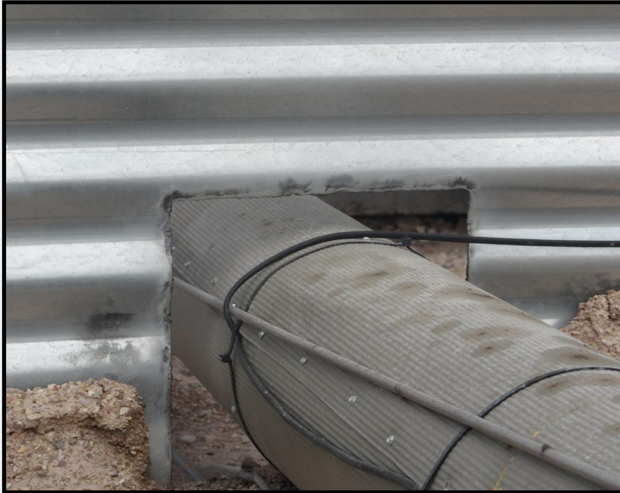
Pipe through secondary containment wall
