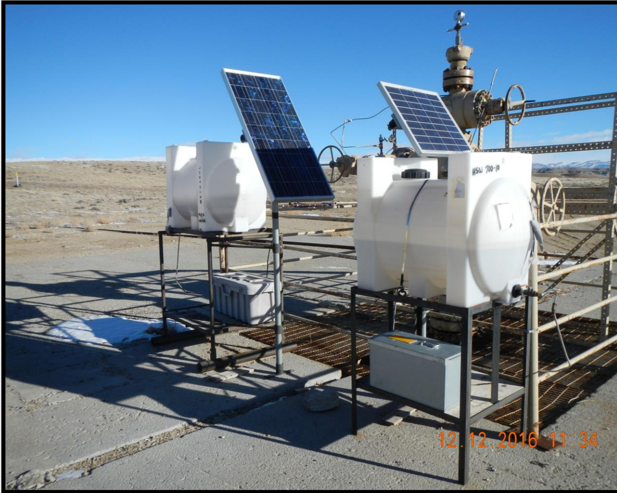
Chemical tanks near wellhead
