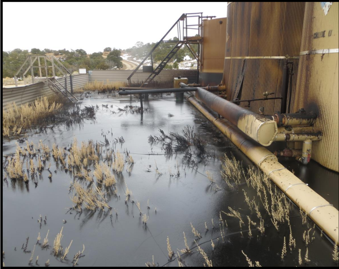
Oil spill discovered within secondary containment
