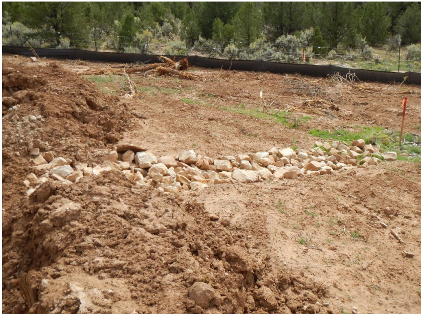
Rock Rundown constructed off SE corner of well pad; Silt fence installed below fill slope of well pad
