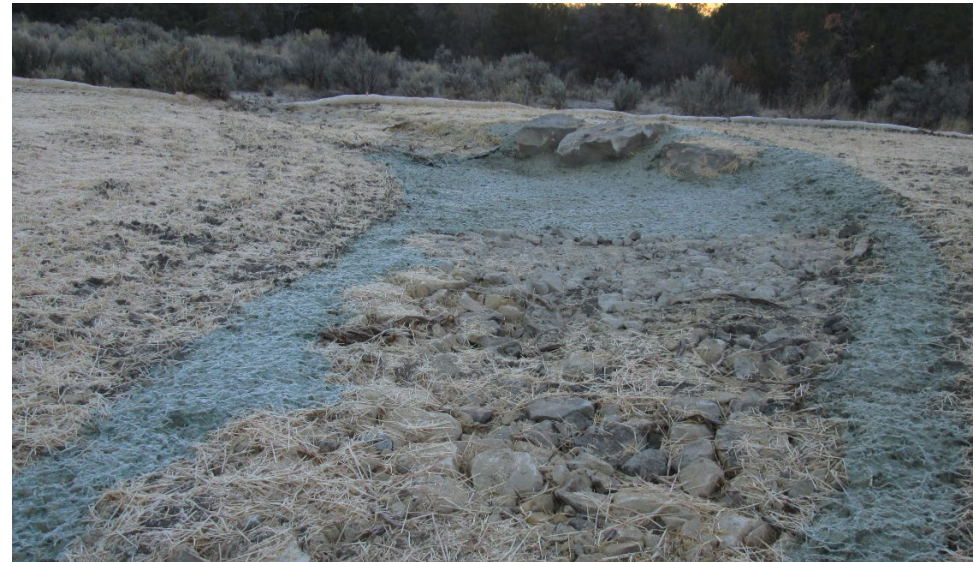
West side of well site seeded and mulched for interim reclamation; Stormwater management outflow off west side of well site
