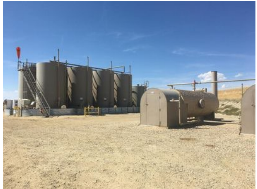
Tank battery within adequate containment structure; All facilities painted Covert Green (complies w/ APD)
