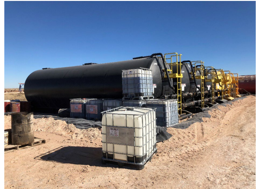
Produced water tanks and chemicals within lined containment; Empty chemical container in foreground
