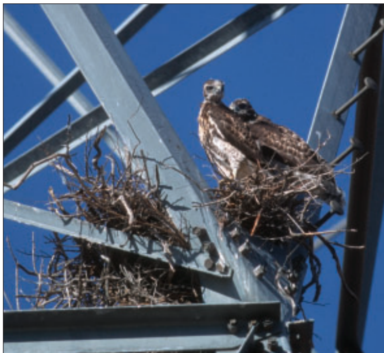
FIGURE 6.3: Red-tailed hawk nest on steel lattice transmission tower.
