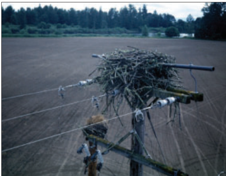
FIGURE 6.23: A segment of plastic pipe was installed on a dead-end pole in Oregon to discourage osprey nesting. However, the osprey pair continued nest construction after the pipe was installed.
