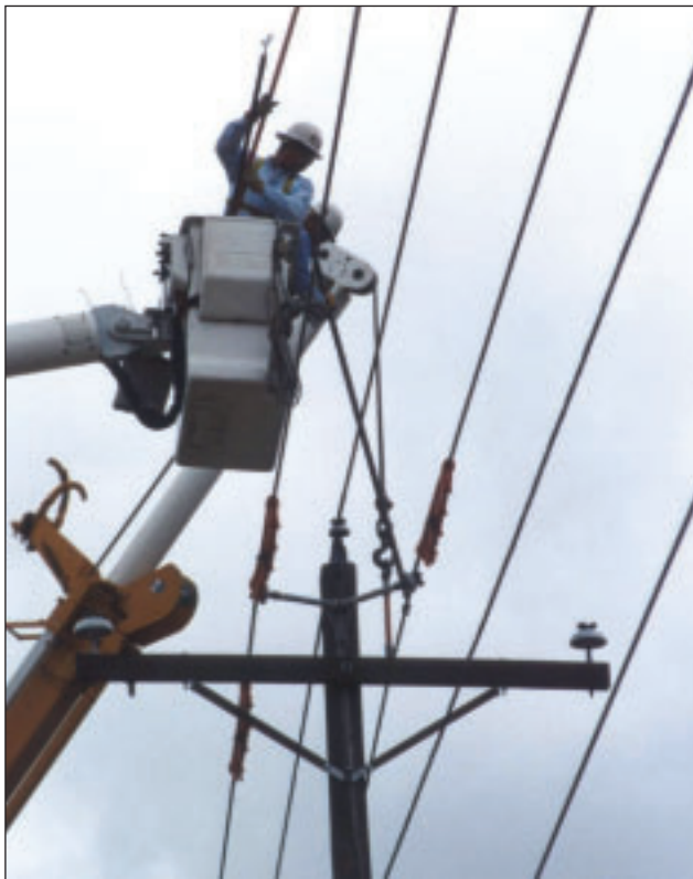
FIGURE 7.2: Reframing a crossarm to prevent avian electrocutions.
