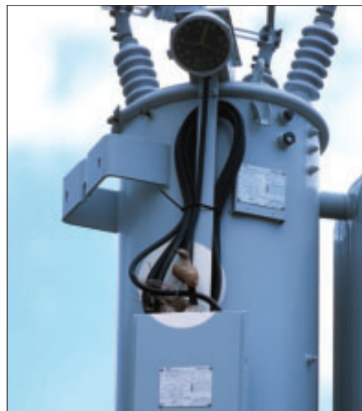
FIGURE 6.7: Western kingbird nest (see highlighted area) on transformer.
