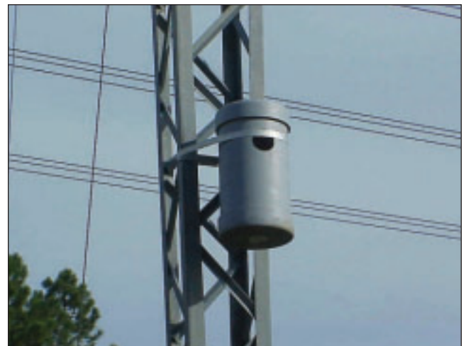
FIGURE 6.20 Kestrel nesting tube (46-cm [18-in] length) installed on transmission tower in Georgia.
