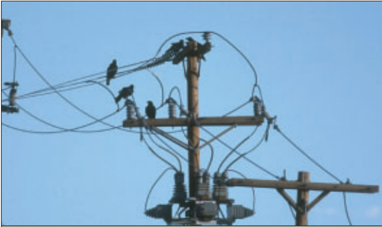
FIGURE 4.15: Numerous birds perched on a pole can increase electrocution risk. Pictured: common ravens during breeding season.
