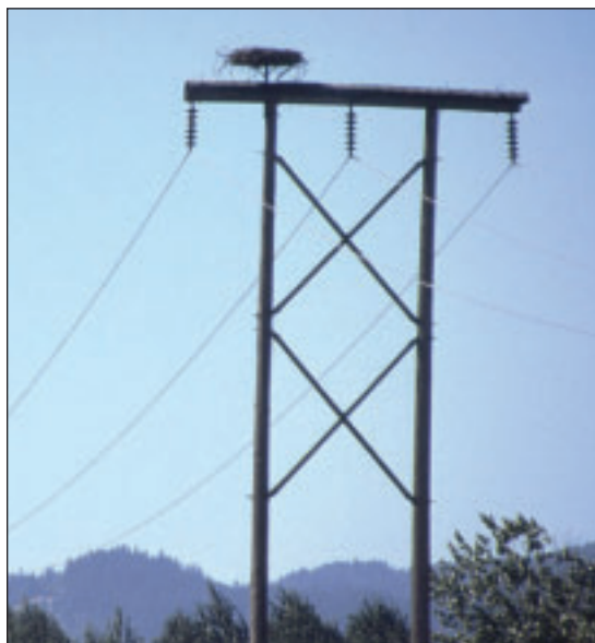
FIGURE 6.22: This osprey nest was originally located on the crossarms above the center conductor where contamination from fallen nest material and excrement accumulated. It was relocated to the platform shown. A halved, corrugated pipe was installed to prevent re-nesting on the crossarms. Relocating a problem nest to a nest platform on an adjacent non-energized pole is preferred. However, if pole cost, rights-of-way restrictions, or limited access prevent installation of a new structure, it is best to install a safe nest platform on the existing structure.
